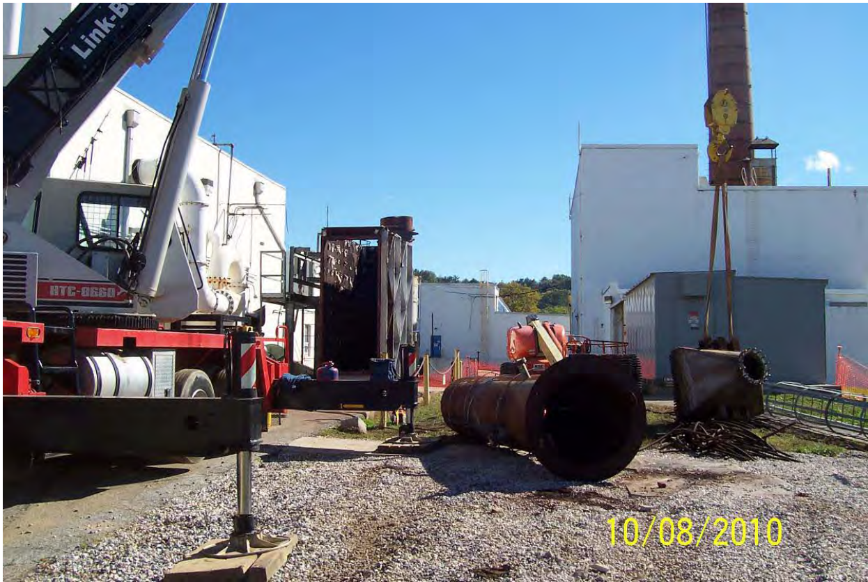
TFO looking east. Both stacks, the recuperator, and the platform was removed.
