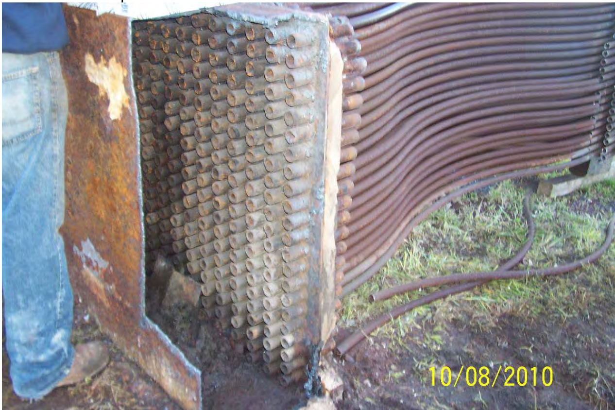
The bottom of the recuperator where the air passed from the carbon steel to the stainless steel rods.
