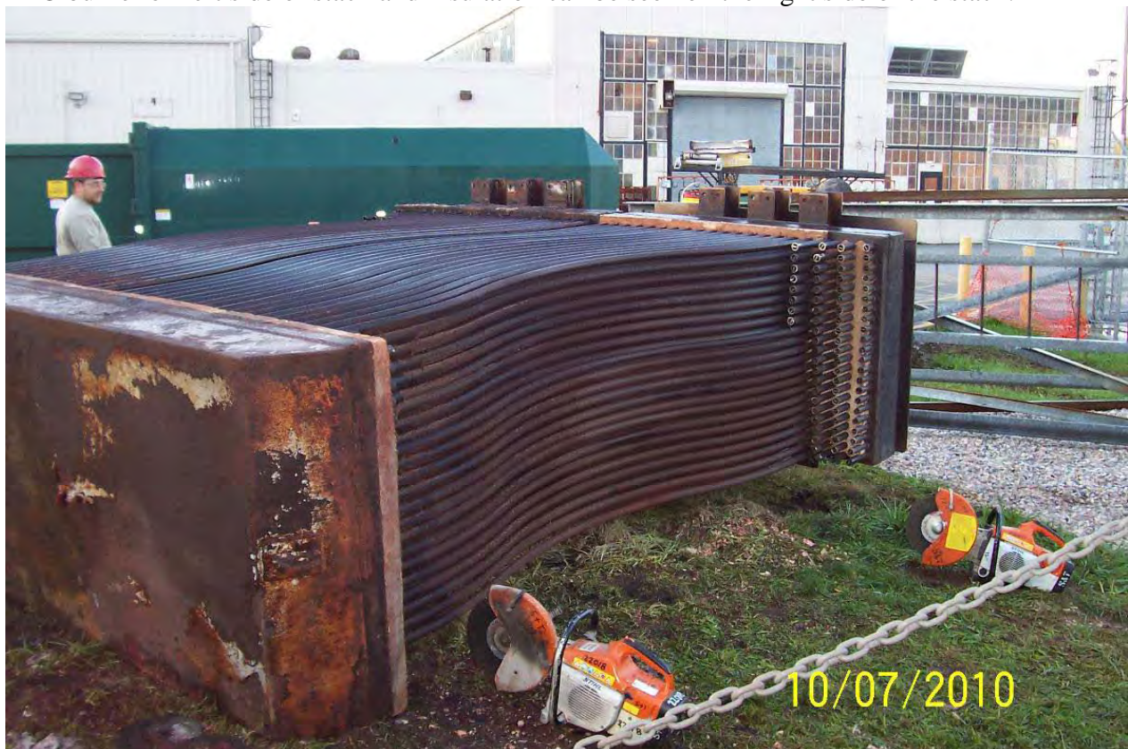
TFO recuperator rods are being removed for scrap. The near side is carbon steel and the far side is stainless steel. These corroded rods restricted air flow through the TFO.
