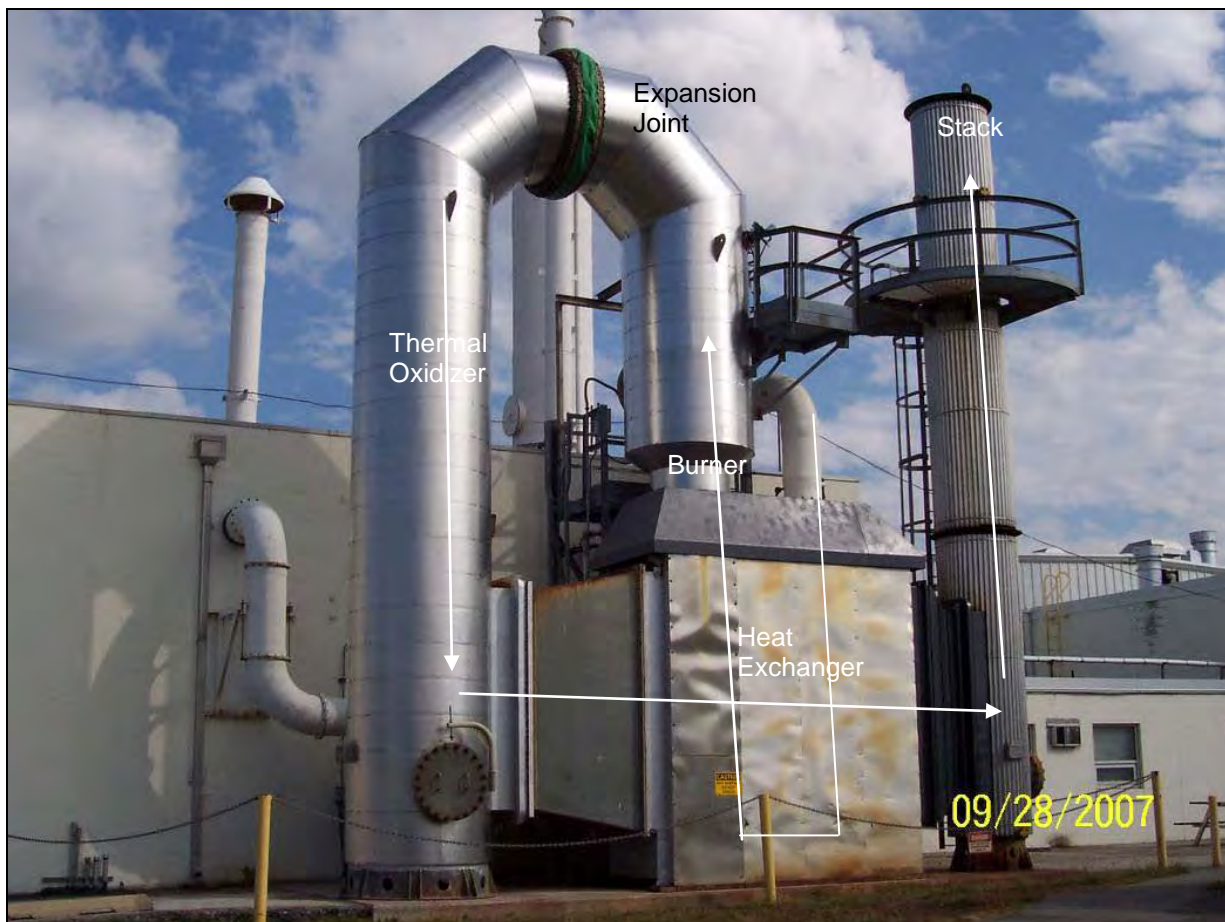
Figure 1. Photo of Thermal Fume Oxidizer before demolition (arrows show direction of off-gas flow).
