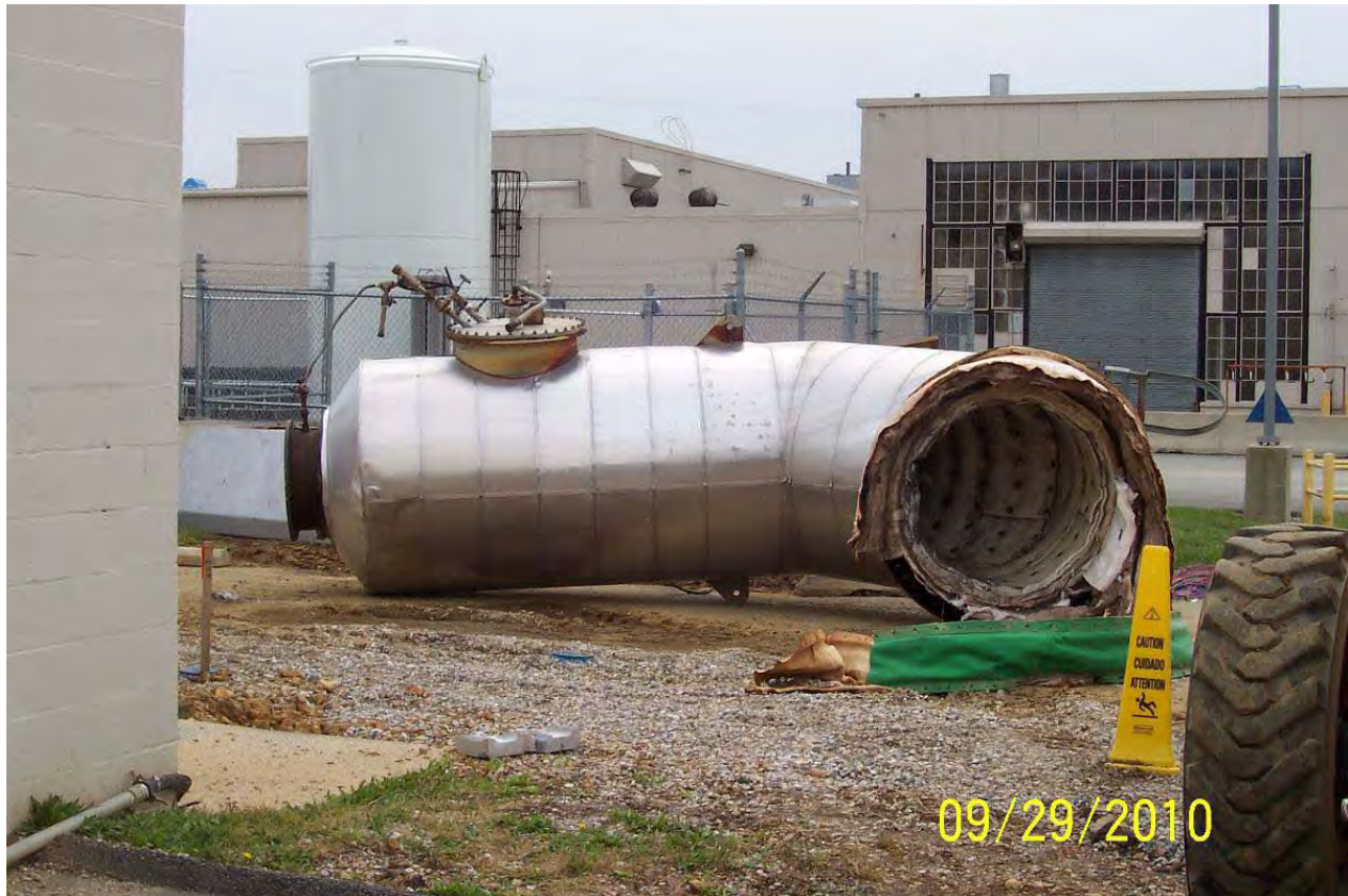
TFO burner on left side of stack and insulation can be seen on the right side of the stack.
