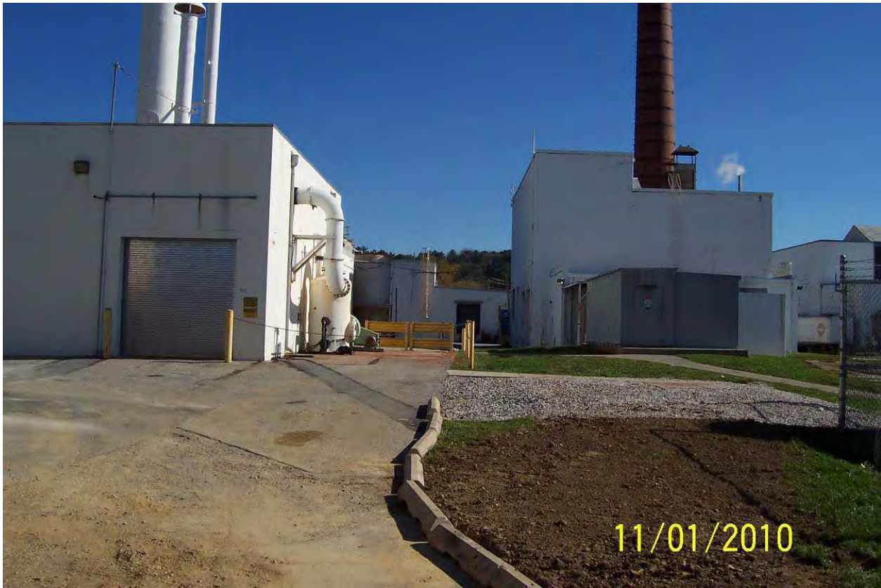
Looking east at the TFO pad after the TFO and hydrogen storage area were removed.
